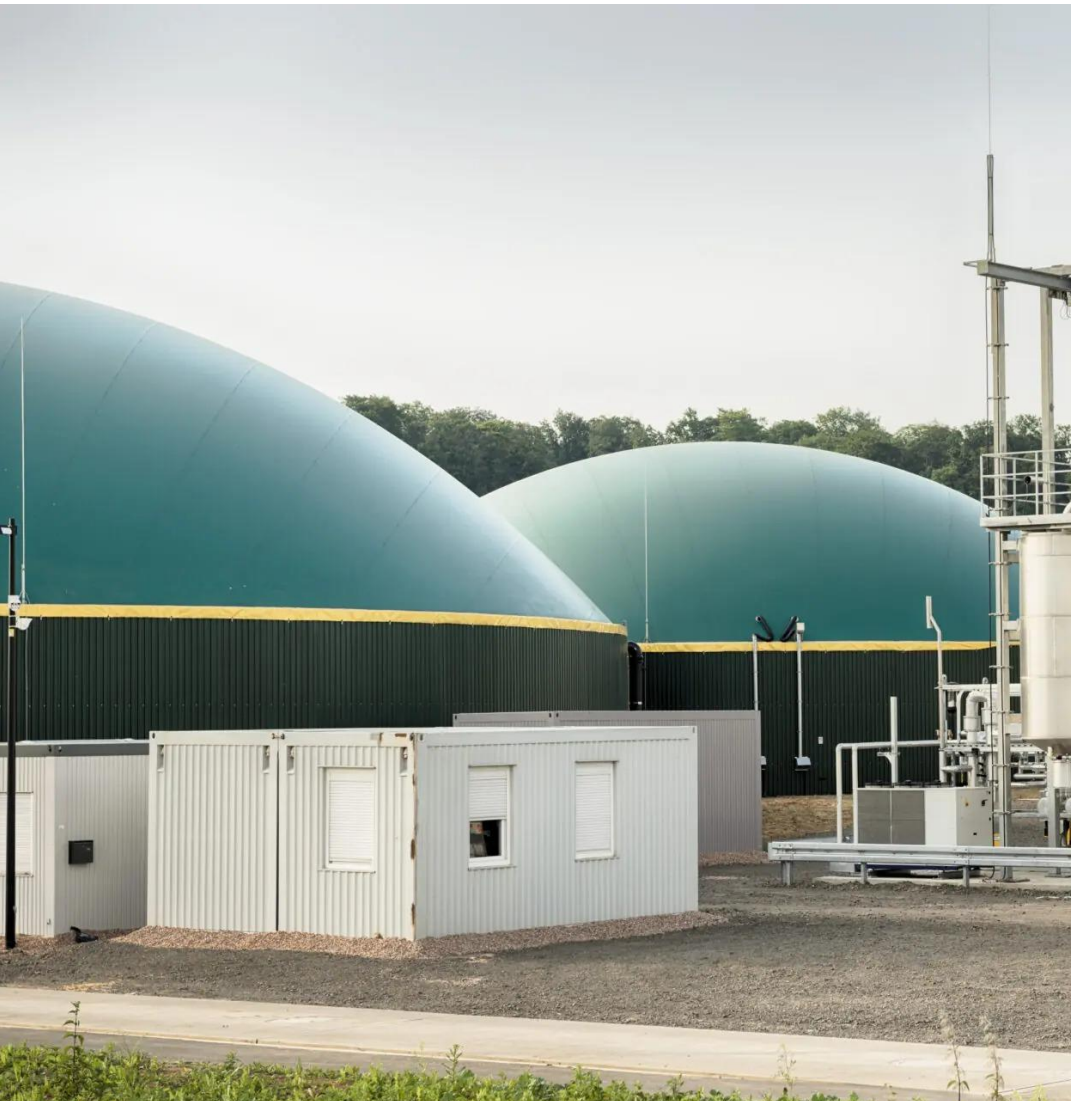
Methanisation unit project, France (CVE Group).
